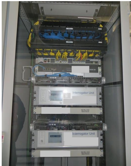
Figure 9 PMS rack mounted equipment at one of the block valve stations
